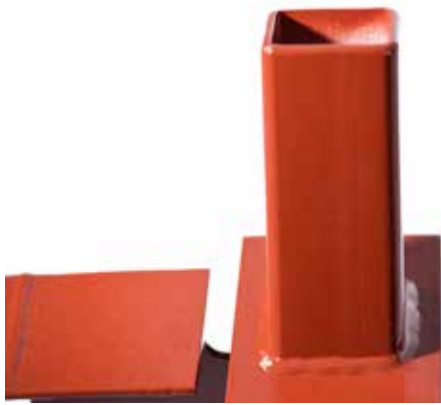
▲ AESS 2: HSS weld seam orientation not defined.
