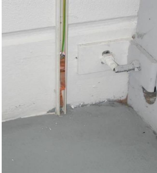
Conventional grounding via “ Conductive copper tape ”
